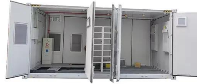
1075KW HH ESS
