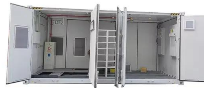
1075KW HH ESS
