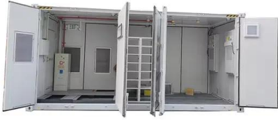
1075KW HH ESS
