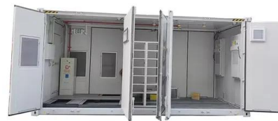
1075KW HH ESS
